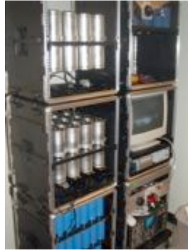
Capacitor bank and instruments
